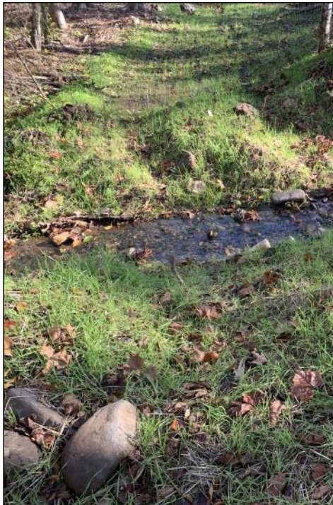
This issue's cover photo is a rehabbed stream crossing in Mitchell County (photo credit: Alan Huskins). Stream crossing approaches can be the leading contributor of sediment on a logging job. Ensuring these sensitive areas are adequately stabilized during and after forest operations helps protect water quality. Grass seed and mulch, used in the picture above, has proven to be an effective BMP in many research studies. Notice that the stream channel is free of debris and only a small amount of bare soil can be found. Nice work!
