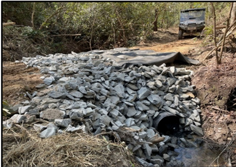
Culvert crossing repair in progress. Headwall has been armored with riprap while additional stone is still needed for the roadway on top of the geotextile fabric.
