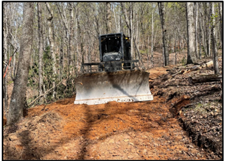
Dozer operator Chris installing water diversions on steep sections of a low standard forest access road that was used as a firebreak.
