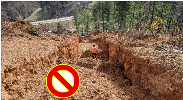
Do not excavate skid trails into the earth!
