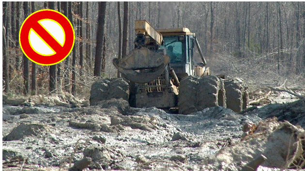
This rutted, soupy skid trail is a risk to water quality and will likely degrade the soil's condition afterwards.
