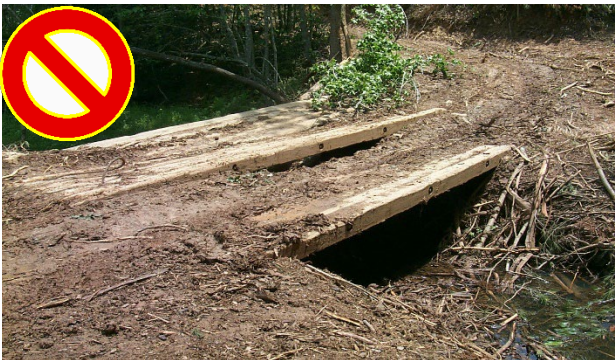
Panels are slipping, soil is entering the stream.
