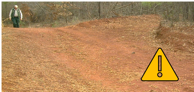
A rolling dip mound at the crest of the road slope diverts runoff into the turnout. Groundcover stabilization is needed.
