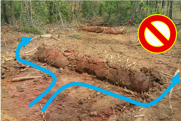
Runoff can easily bypass around both ends.
