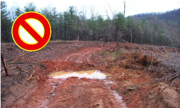
Waterbars should not collect water and an outlet is needed.
