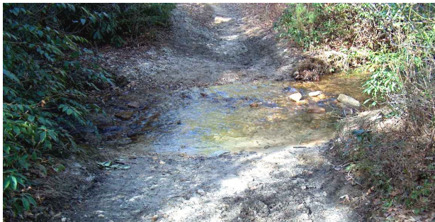
BEFORE: Bare soil and no hardening of the crossing.
