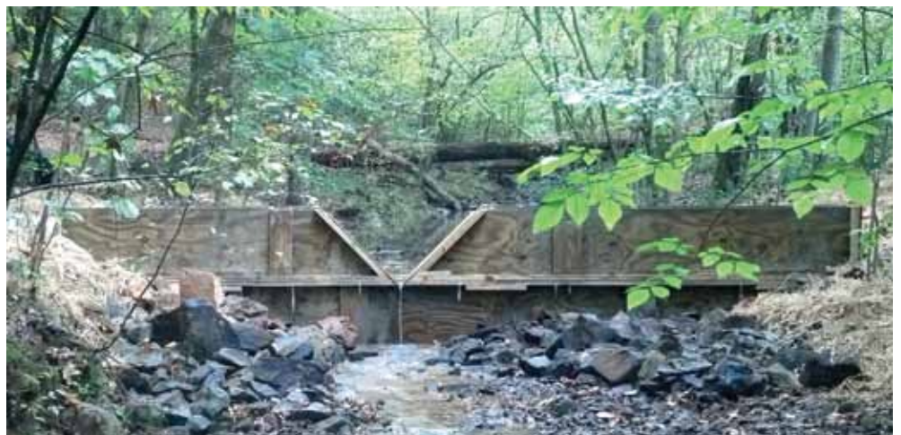
Temporary stream gages are installed to calibrate the stream flow, so that precise measurements of sediment in the stream can be obtained. The stream above was temporarily pumped around this site during installation. Upon conclusion of the study, the gage structure is removed.
