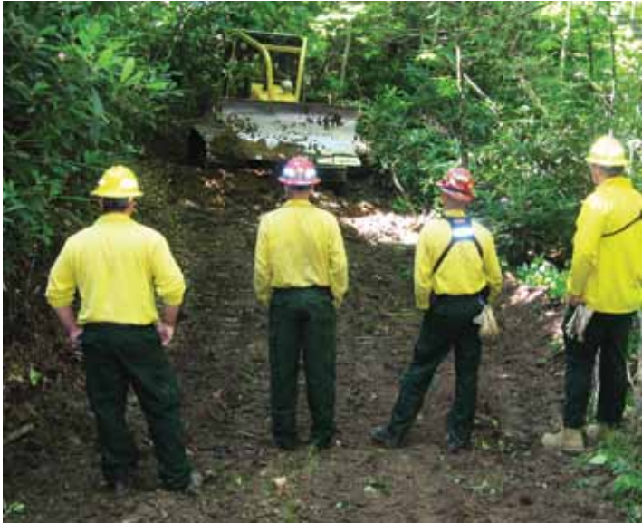
A team of NCFS operators watches while another team member prepares to install a waterbar runoff diversion on a trail at Gill State Forest in Avery County
