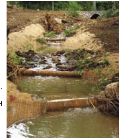
Upstream view of newly-installed culvert, log veins and rootwads a few days after installation.
