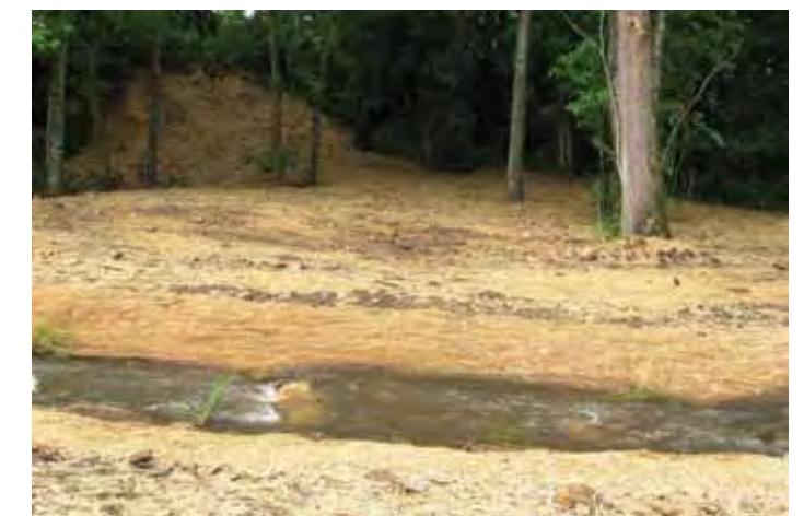
AFTER, May 2009: A new, appropriately-sized stream channel was established away from the embankment, seen in the background after soil and straw had been applied for stabilization. This view of the new stream is less than one week after completion, during which the site received nearly three-inches of rain.
