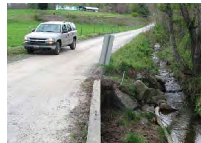
BEFORE, April 2009: Purlear Creek was situated alongside Mozelles Road and was functioning as a drainage ditch. Sediment could easily wash into the stream.
