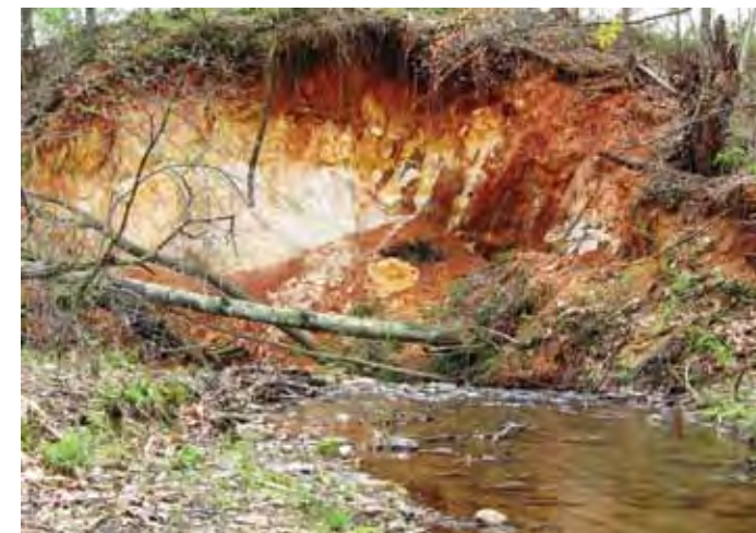
BEFORE, April 2009: Purlear Creek flowed along the base of this collapsing embankment that supports a public road (SR1350, Mozelles Road). Relocating the stream kept sediment from getting into the water and eliminated an ongoing threat to the road's sub-structure.
